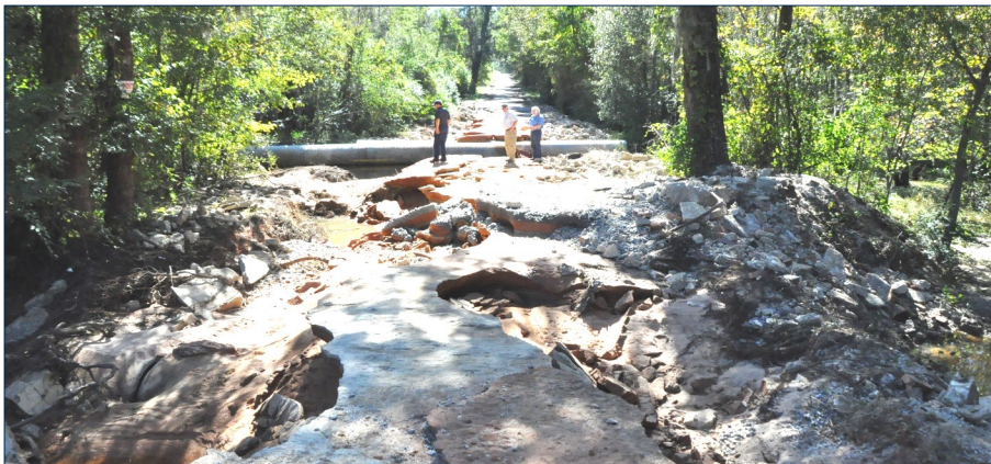
SCEMD recovery specialists conduct a site visit in Florence County to inspect damage caused by Hurricane Matthew.
